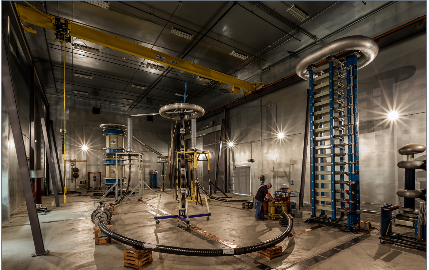
▲ G&W high voltage testing laboratory in Bolingbrook, IL
