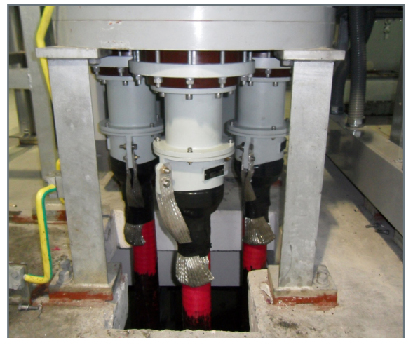
▲ SSC140-SF terminations installed in a GIS.
