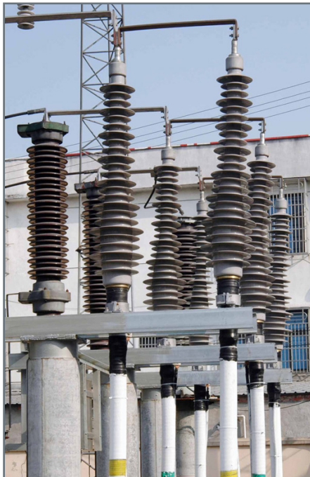
▲ Dry type outdoor termination in a substation application.
