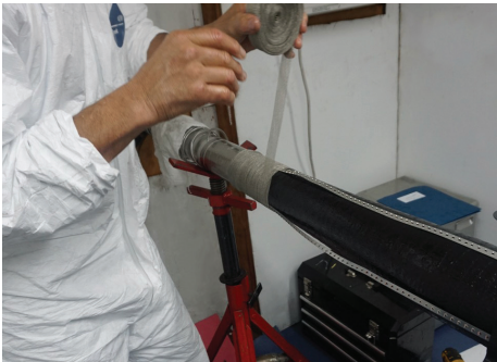
Application of the tinned copper braid over the ground electrode of the joint.
