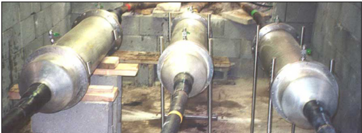
Splicing each leg of the three phase cable permitted a low profile, shallower vault.
