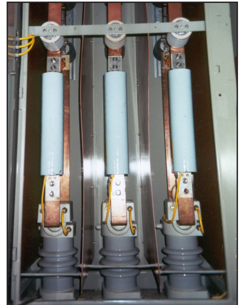
15kV CLiP fuses mounted in an enclosure.
